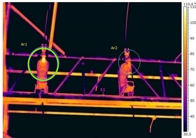
Figure 3.5 Infrared image of substation disconnects
