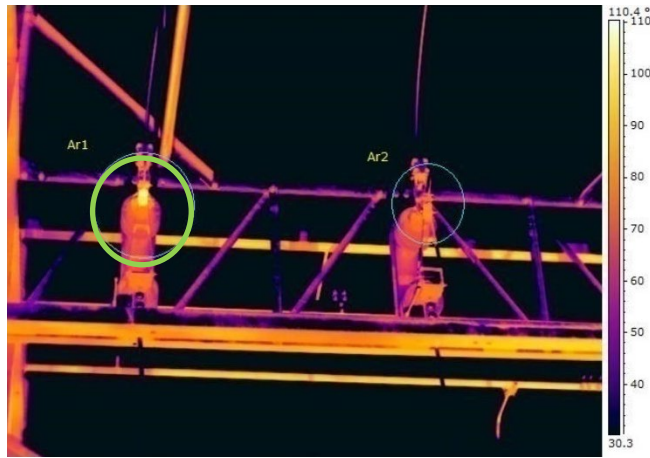
Figure 3.5 Infrared image of substation disconnects
