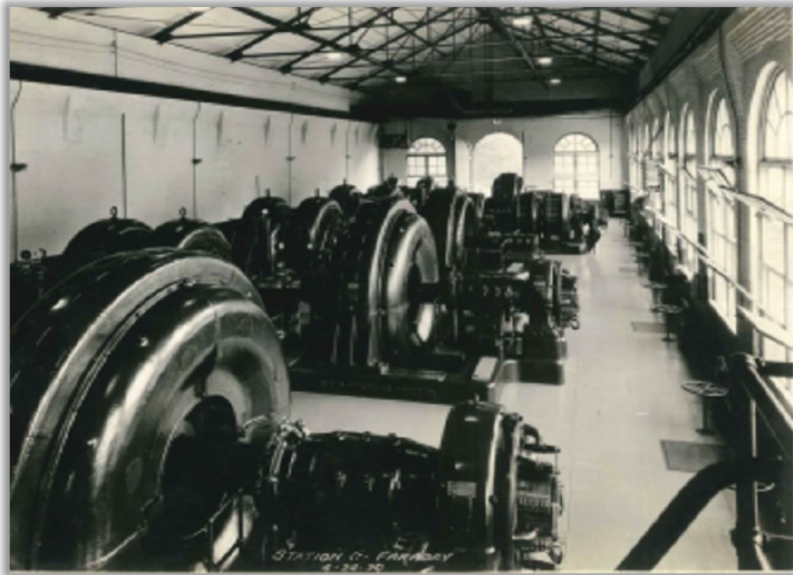
Figure 2 1907 Faraday Powerhouse Interior
